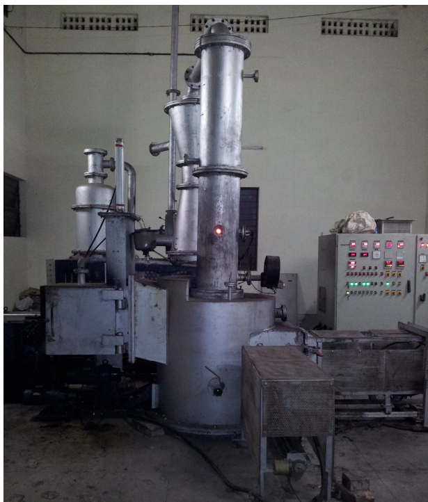
Fig. 1: Plasma Pyrolysis system installed at Trivandrum
