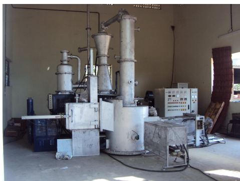
Fig. 1: Plasma Pyrolysis system installed in Trivandrum
