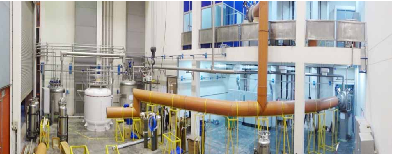
Figure B.2.4 Prototype Cryoline (PTCL) Test Infrastructure at ITER-India lab
