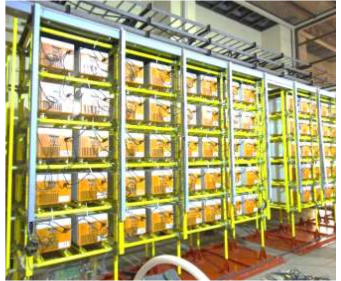
2.5 MW, 100kV HVPS operational at LEHIPA facility, BARC
