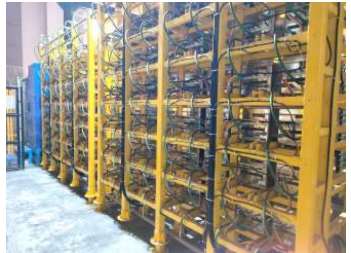
6MW, 55kV HVPS operational at ITER-India, IPR
