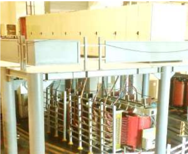
3 MW, 27/18kV HVPS operational at ITER-India, IPR
