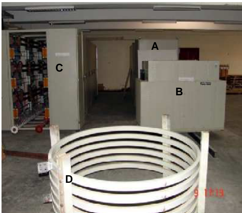
IGBT-based Inverter Power Supply for SST1 Plasma Vertical Position Control. (A) SCR Controlled AC/DC Converter with Filter Choke. (B) Dry type converter transformer. (C) IGBT-based DC/AC Inverter Stacks. (D) Water cooled inductive test load.
