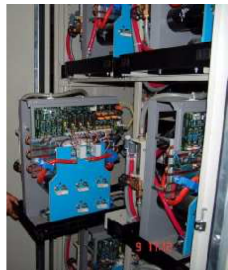
Individual module of the inverter stack –One of the 72 modules, retracted out for access - Each module includes DC CAPs, IGBT Inverter, Embedded Digital Controller with Ethernet.
